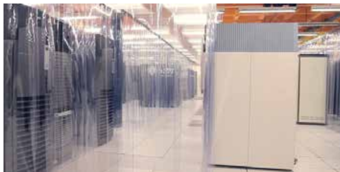
Energy optimisation - Vodaphone Datacentre France
